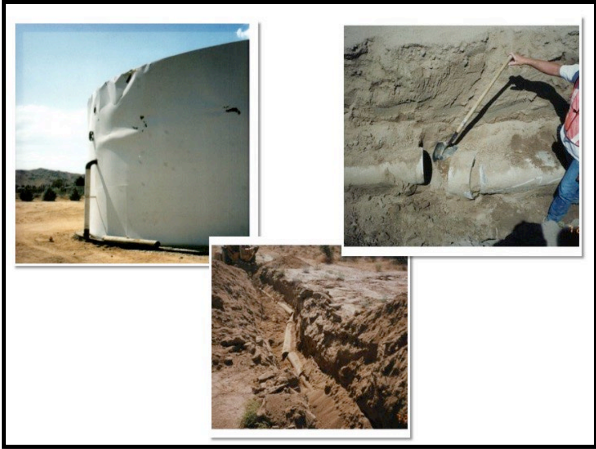
Figure 2 Examples of Earthquake Damage to Water Utility Facilities These examples were from the 1992 Landers Earthquake
