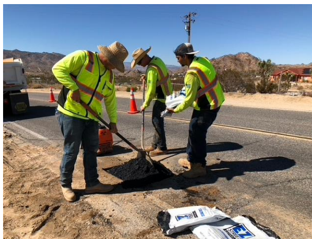
Photo Caption: Team work! Just another day and another leak that required half a dozen crew members, and numerous pieces of large equipment to make repairs quickly on our ever aging old pipe system. This was the Quail Springs Road leak.
