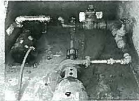
Caption: Existing Piping Configuration
