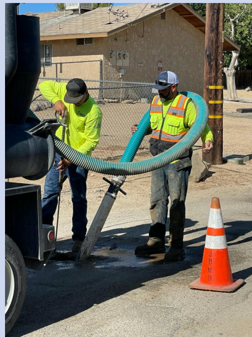
Photo Caption: JBWD crews fixing a leak using a vacuum to excavate down so no other utilities in the
