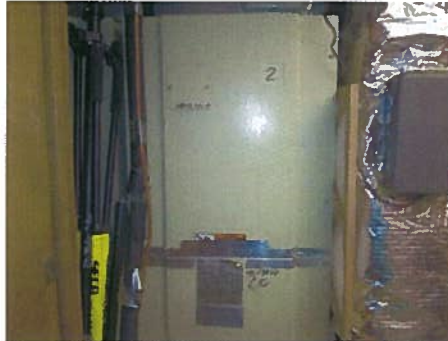
Photo 6.0 Existing FCU-2 serves Board Room & Copy/IT Room located in Hallway Closet (similar for FCU-1 and 3)
