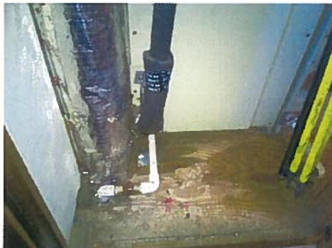
Photo 7.0 Existing FCU-1, 2, and 3 Closet Return Air Plenums with possible moisture damage from condensate drains)
