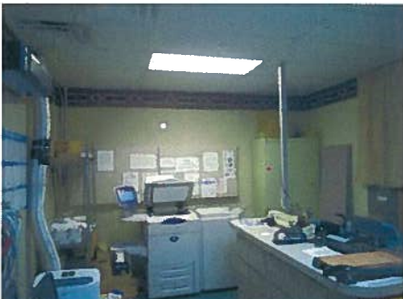
Photo 11.0 Existing Copier Room with IT/SERVER unit, and spot cooling "LG" ductless unit. This zone is also served by FCU-2 that serves Board Room
