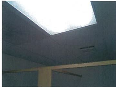
Photo 13.0 Existing Men's Toilet Fan (appears undersized)
