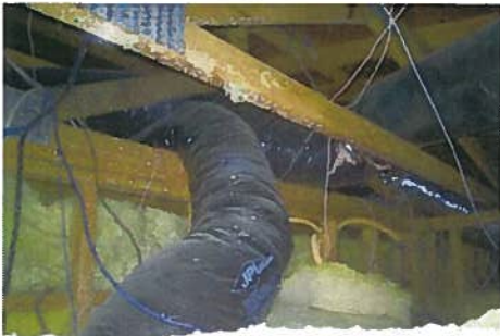
Photo 2.0 Existing Flexible Ductwork in Attic (typical throughout building, creates poor airflows)
