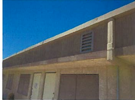
Photo 12.0 Existing Attic Space Fan, and outdoor Soffit Intake louver, recommend to upgrade
