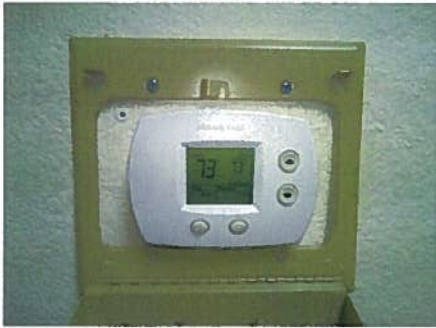
Photo 9.0 Existing Thermostat (Typical)
