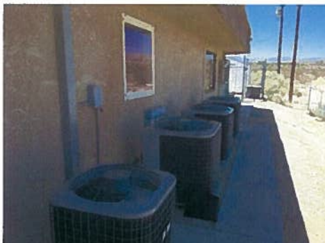
Photo 8.0 Existing (4) Outdoor Condensing Units
