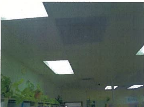
Photo 3.0 Existing Typical Ceiling Grid & Grilles
